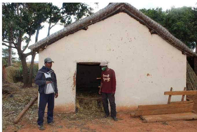
Picture 11 : Improvement of a stable with a grant from the project in Inanantonana
